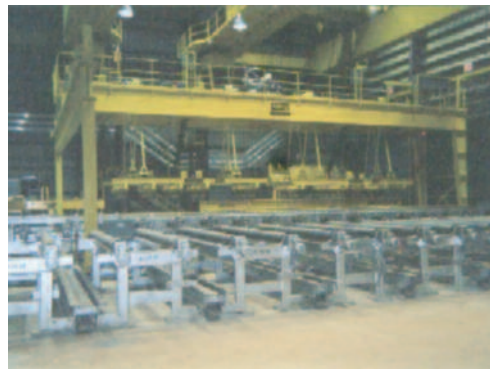
Overall View of the Semi-Gantry Plate Loader
